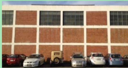
A cavity brick wall. Many walls of this type are often plastered over on our Art Deco buildings so they are not obvious to the casual observer
